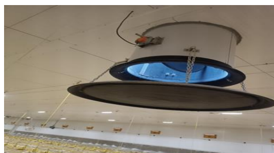
Figure 2 – Exhaust ventilation shaft mounted on the roof, with flap
