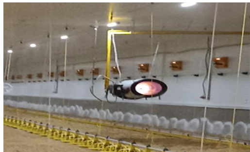
Figure 4 – Gas air heater
