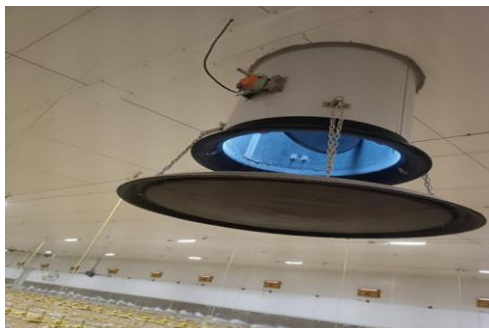
Figure 3 – Exhaust ventilation shaft mounted on the roof, with flap
